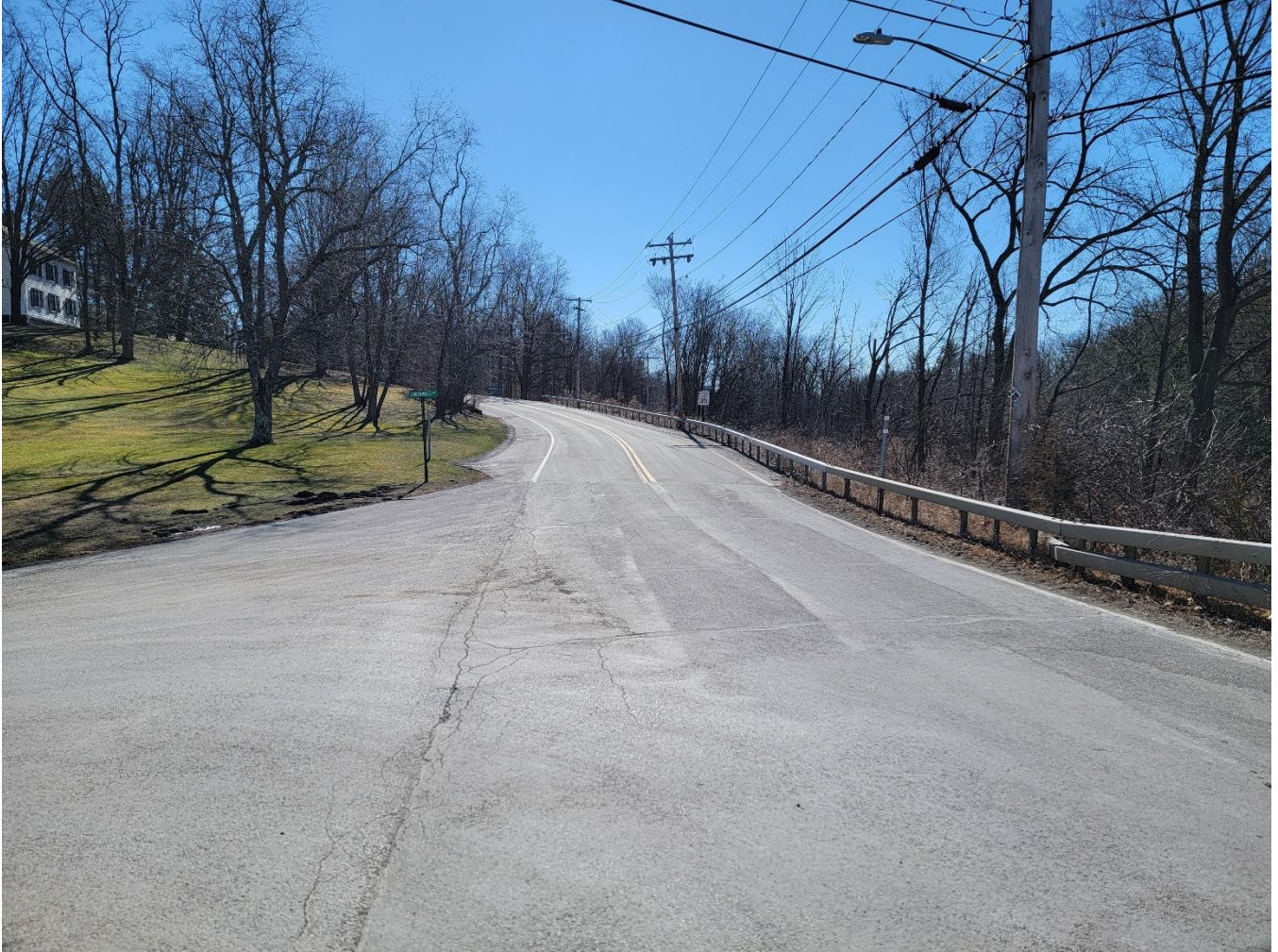
Photo 12: Looking south at the intersection of County Route 25A and Lindenwald Avenue
